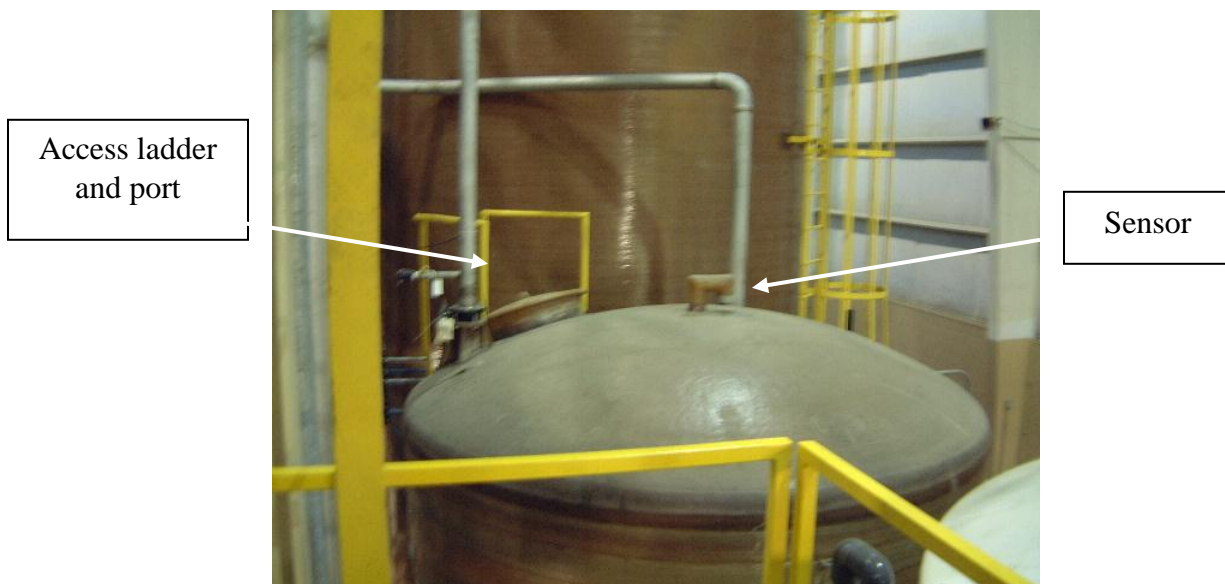
Figure 3 Storage tank without safe means to access sensor
